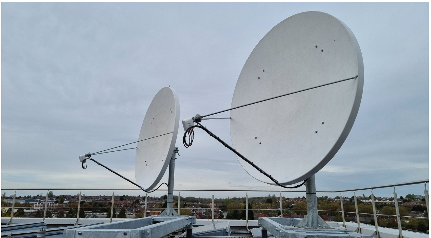
Dartcom Ku-Band EUMETCast System with additional antenna aligned on the Europe backup satellite to provide higher availability
