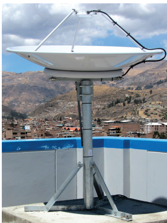
Dartcom GOES HRIT antenna installed at the University of Huaraz in Peru
