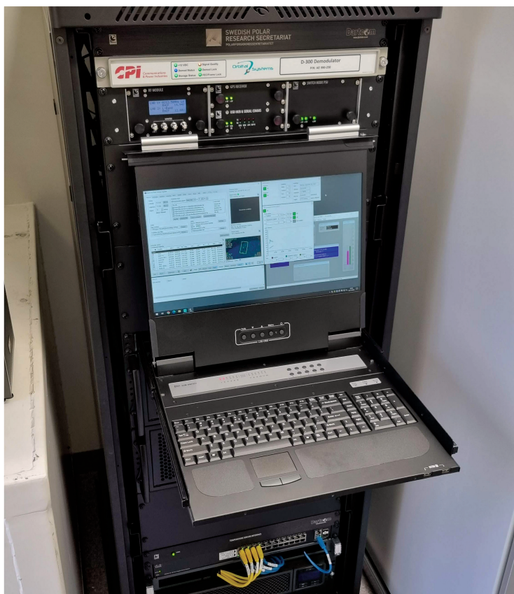
Floor-standing equipment cabinet with rack-mount PCs and KVM console
