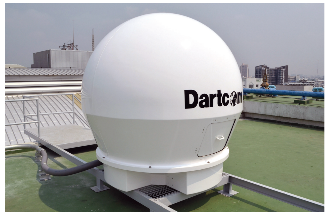
Dartcom X/L-Band EOS System at Chulabhorn Satellite Receiving Station, Kasetsart University in Bangkok, Thailand
